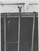
TANK PLATES are cut away from the structure before a tractor is called in for the "tangerine peeling" operation.
